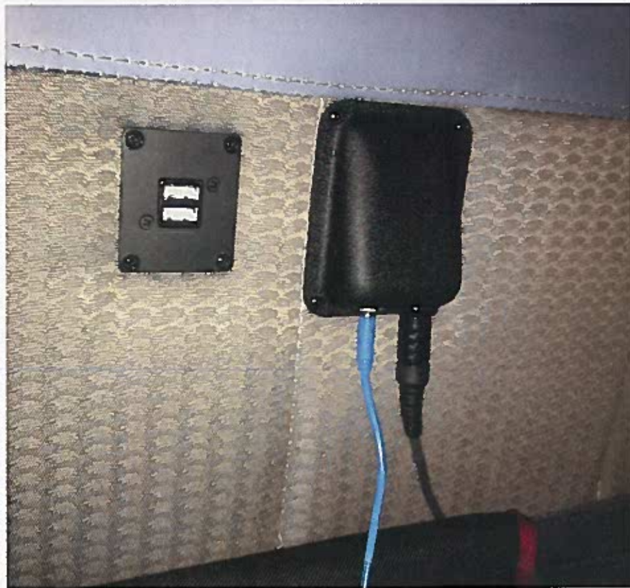
Mid-Continent True Blue Power TA102 USB Charging Port mounted on the sidewall in the back seat. Note the added port for portable audio which may be used when the back seat passengers are isolated from the "crew" on the audio panel. A similar installation (without the audio port) is on the opposite aft sidewall.
